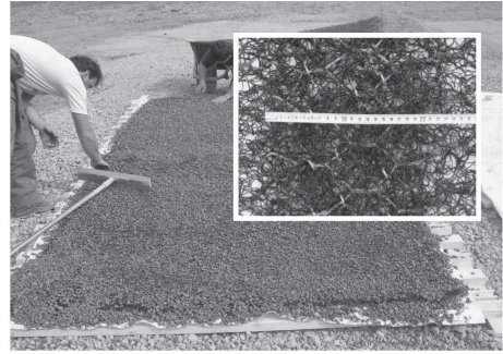
Figure 3. The filter mattress ballasted with the 4-8 mm gravel, together with a detail of the PP geomat reinforced with the wire mesh.
