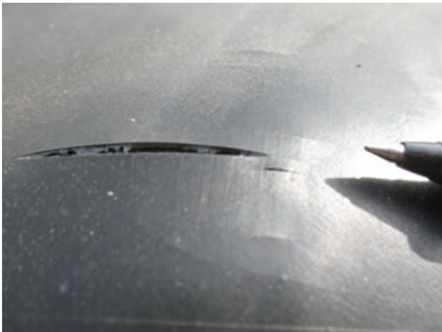
Figure 1. Typical SCG cracks on extrusion die marks at subgrade stone protrusion
