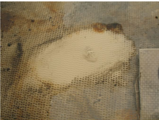
Figure 7. Short cracks (circled) at ballast tube end protrusions
