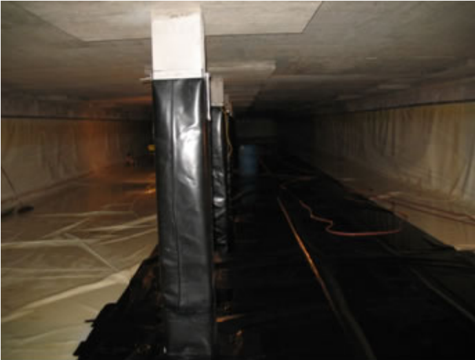
Figure 9. Potable water reservoir liner
