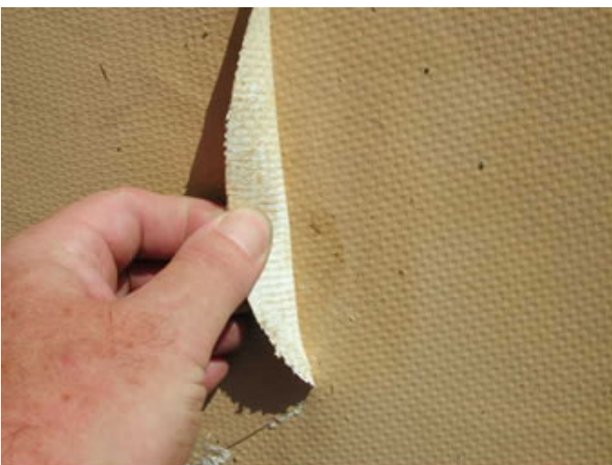
Figure 8. Poorly bonded repair patch
