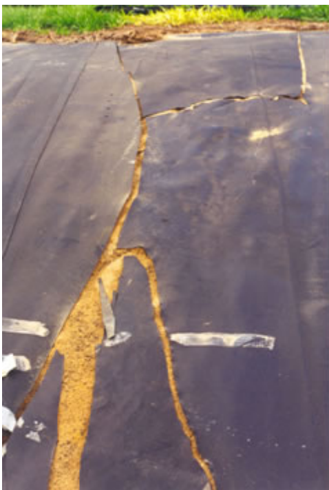
Figure 2. Crack along edge of weld moving into panel of fPP
