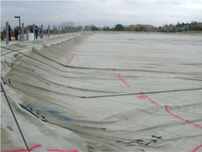
Figure 6. Cracking (dark areas) in tensioned fpp-R floating cover
