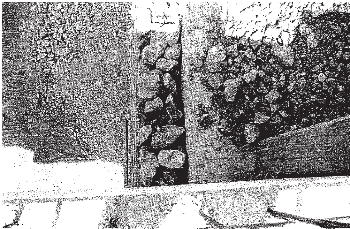
Figure 4. Looking down on front of bridge seat. Note clearance behind wire facing, top of precast panel walls below. Bridge deck is in foreground.
