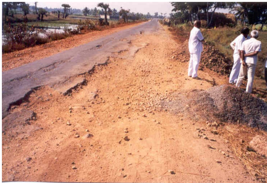
Figure 8. The canal road under severe distress
