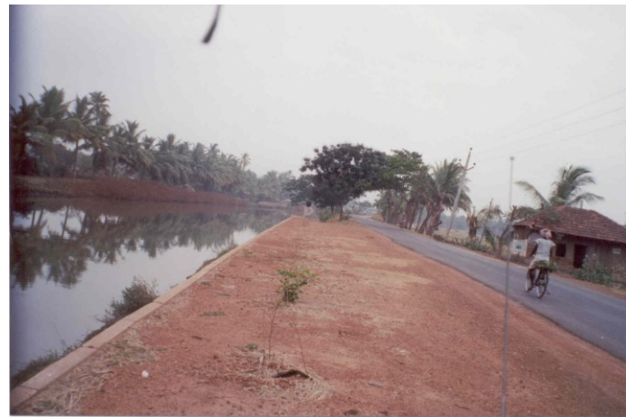
GEOSYNTHETIC REINFORCED SOIL WALL WITH GEOCELL MATTRESS – Marteru – Prartilanka Road, A.P. (Tensar Geogrids – Precast Concrete Facia)
