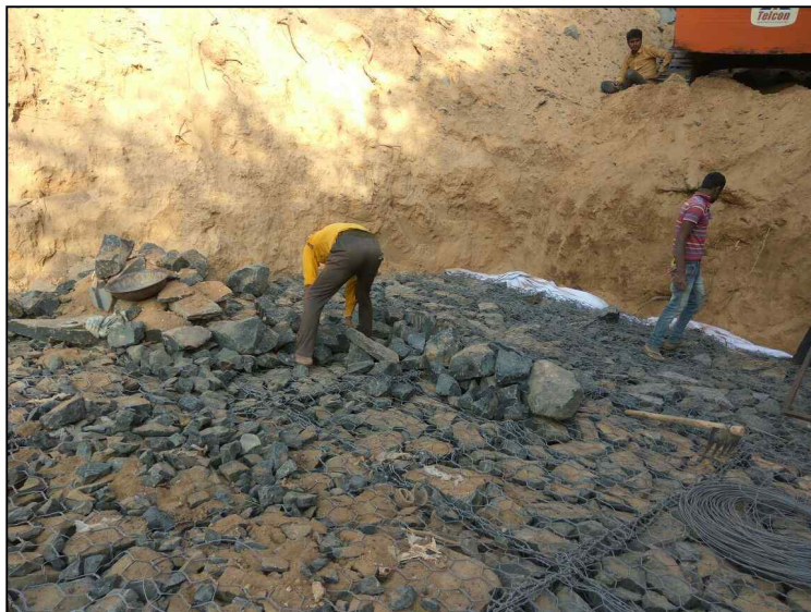
Figure 4: Placement of apron at the toe of wall and lacing of the gabion sheets
