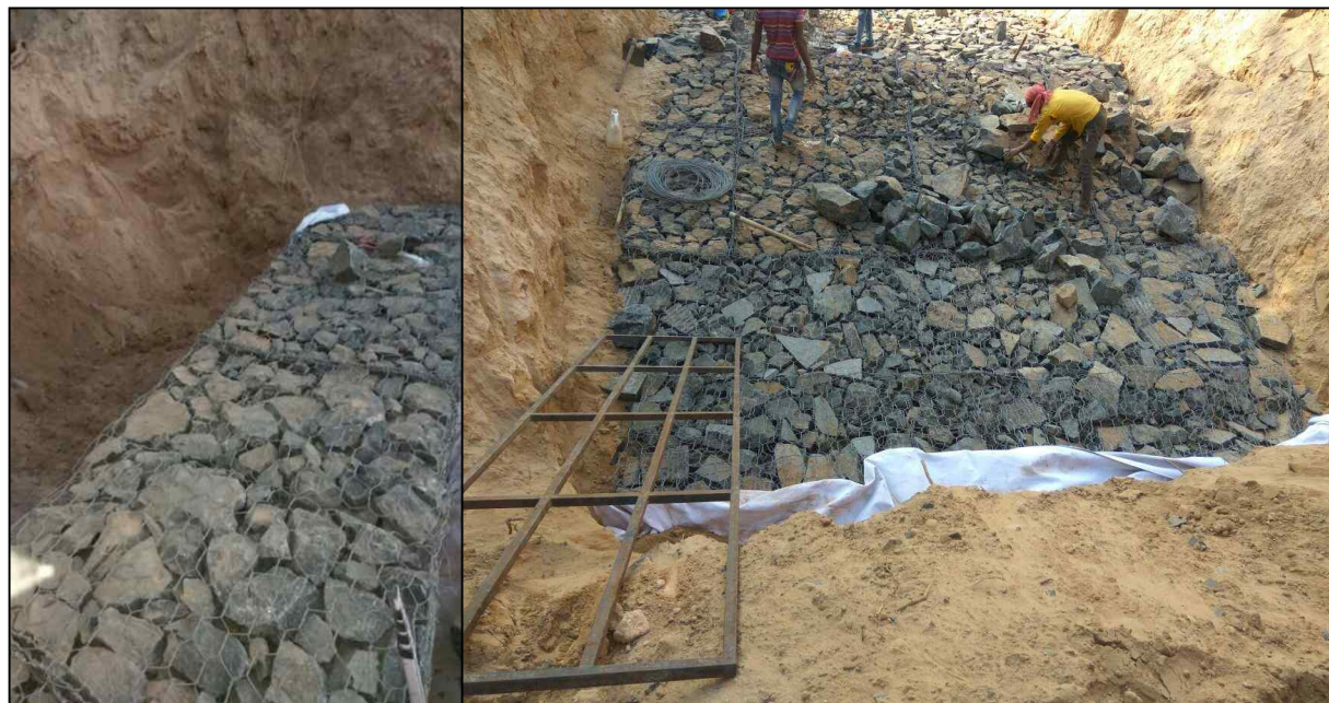
Figure 6: Lacing of adjacent gabion boxes and placing them by providing required offset
