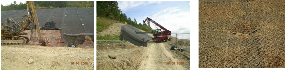
Figure 12...14: construction moments in a slope of mudstone; in figure 12..13 the surface starts to cover with the erosion protection mat
