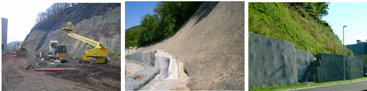
Figure 8...10: Construction moments and the growing vegetation over a time period of 8 months
