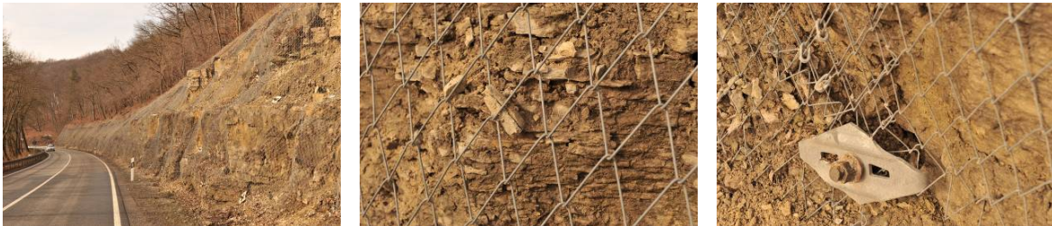
Figure 16...18. A bad example: Details of slope retaining in Muschelkalk WITHOUT erosion protection 6 months after completion
