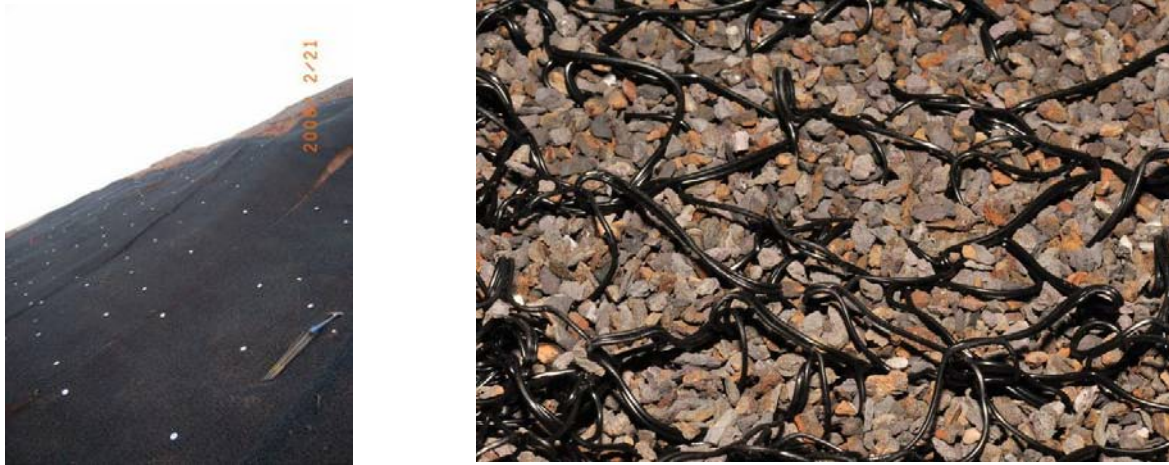
Figure 20...21: Claw mat placed on the slope (unfilled) and a filled with crushed grains of size 1 to 3 mm
