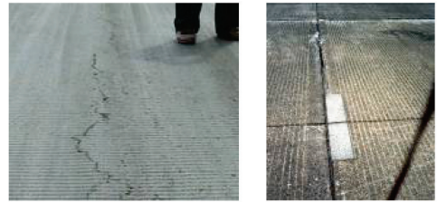
Figure 4. Fatigue cracking of asphalt concrete pavement and spalling and disintegration of joint sealer at concrete pavement.
