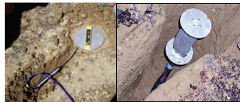
Figure 2. Load-associated instruments include (a) Pressure cells and (b) LVDTs.
