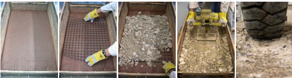
Figure 2. Photographs of test sequence. From left to right - clay subgrade, geogrid placement, sub-base addition, sub-base compaction and trafficking.
