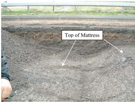
Figure 7. Uneven top of geogrid mattress.
