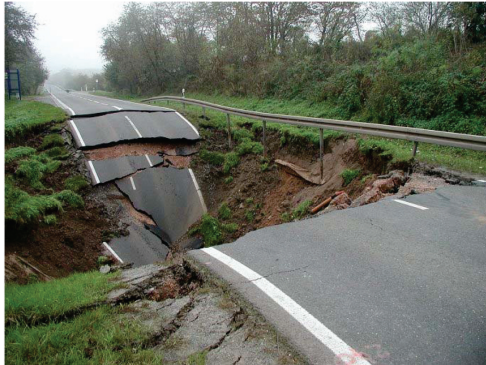
Figure 2. Sinkhole in an existing highway, caused by dissolving of water-soluble stones (B 180, near Eisleben).
