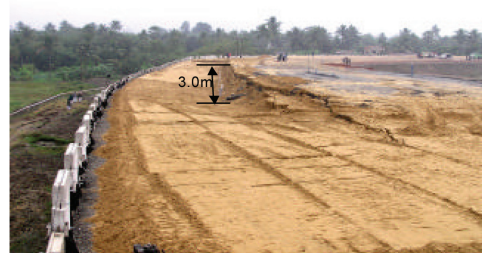
Photo 2. Slip circle failure during Stage-III construction at Km: 26.1 Loop, Kona Expressway, WB-I (Ch. 760 m to 870 m).
