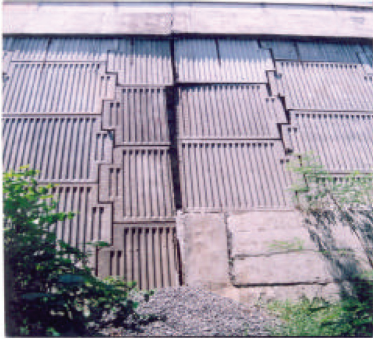
Photo 3. Opening of slip joint at interfaces of reinforced concrete reinforced concrete culvert and reinforced concrete wall.
