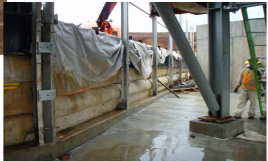
Figure 4. The lower portion of the wall ready for facing panel installation – Note: geotextile ready to be wrapped around.
