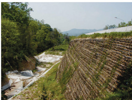
Figure 2. The picture of reinforced slope Lamphun – Lumpang highway with its height over fourteen meters.
