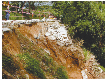
Figure 1. Type of side slope failure at Doi-Tung, Chiang Rai Province, Thailand.
