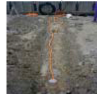
Photo-9 Earth pressure meter in reinforced earth bottom
