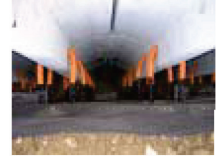
Photo-5 Absorption layer for deformation (before input of crushed stone/View from top down)
