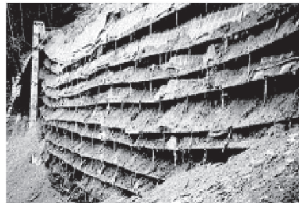
Photo-1 Example of collapse of reinforced retaining wall.
