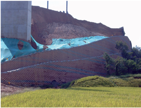
Figure 2. Photo of collapse in the reinforced soil wall.
