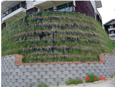
(b) Hybrid reinforcement (After grass germination)
