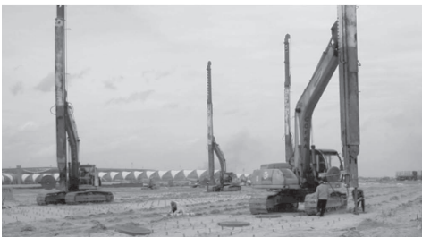
Figure 10. Installation of prefabricated vertical drains at New Bangkok International Airport Project, phase 2.
