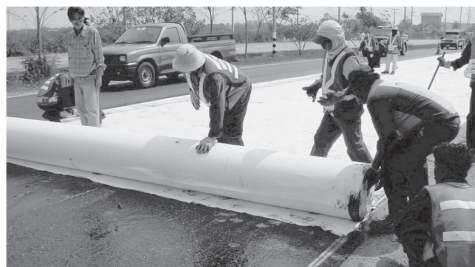
Figure 7. Laying of paving geotextile in pavement overlay work for Minburi to Chachoengsao Road Rehabilitation Project.
