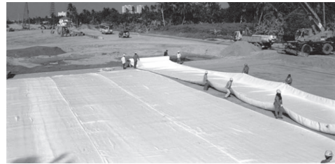
Figure 4. Laying of high strength woven polyester geotextile at Wat Nakorn-In Project, contract EW1.
