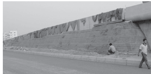
Figure 5. Geogrid reinforced steep embankment side slope at Wat Nakorn-In Project, contract EW1.
