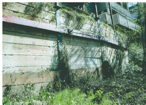
Figure 5. Existing anchored retaining wall system after nearly six years.
