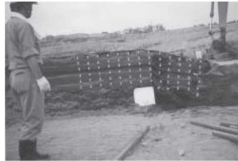
Photo 1. Overview of soil cantilever of type A when its span length reached 1.5 m.
