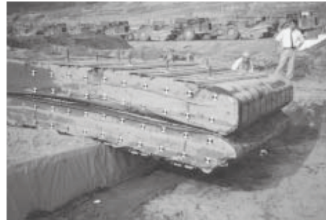
Photo 2. Overview of soil cantilever of type B when its span length reached 1.5 m.
