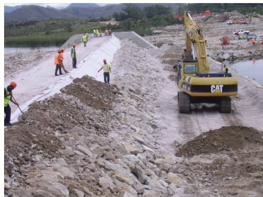
Figure 15. Final stages of the embankment construction showing the above water level sand core, geotextile, filter, rockfill and riprap layers
