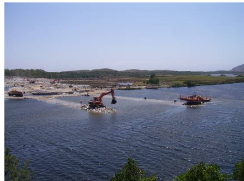
Figure 11. The two pioneer rockfill embankments as they progress across the river just below water level
