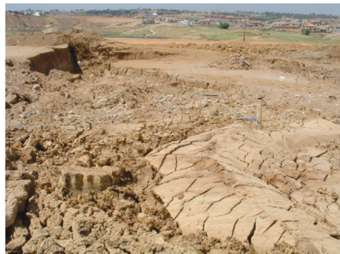
Figure 5. Cover material sheared.
