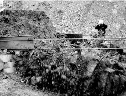
(c) Situation after the failure
