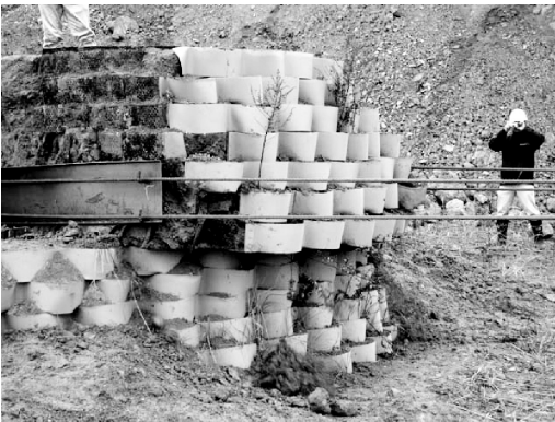
(b) Situation at the failure
