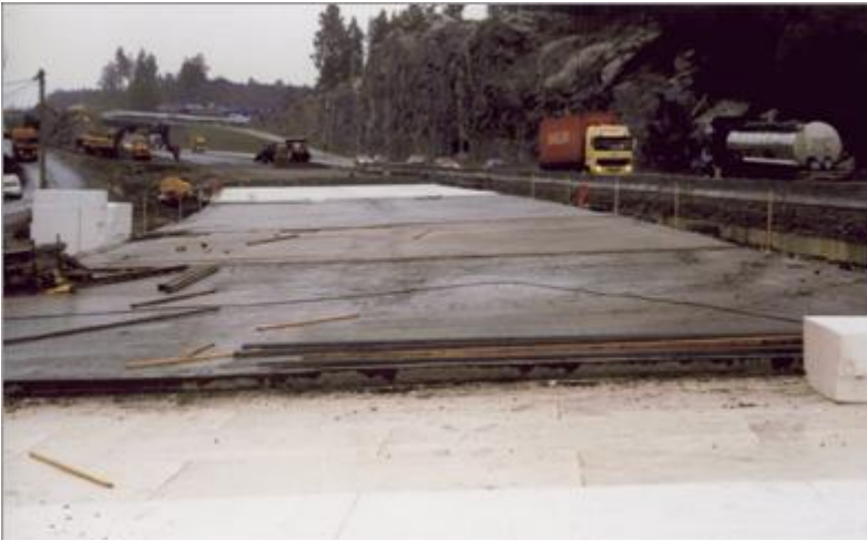
Figure 6. Example of light-weight structure with concrete course above EPS blocks with longitudinal profile and crossfall.
