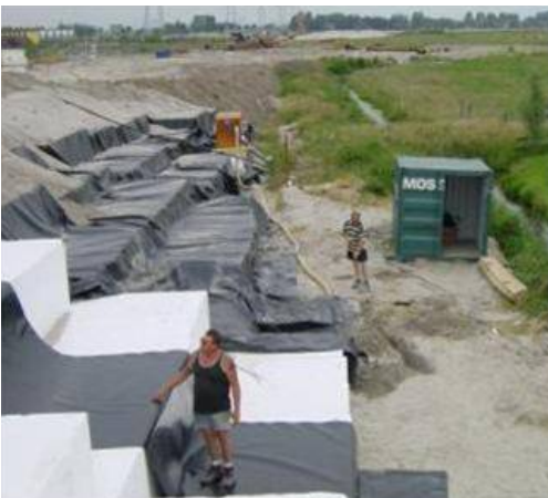
Figure 5. Example of the protection of EPS blocks on the embankment side with HDPE impermeable foil
