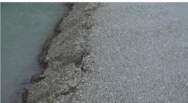
Figure 12. Surface erosion in the SM01F15d section
