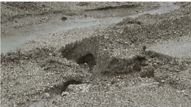
Figure 11. Surface erosion in the unreinforced section
