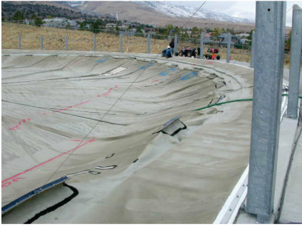
Figure 3. Cover tensioned directly to top of post rather than via pulley at base of post.
