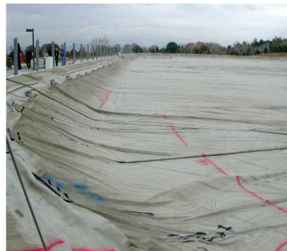
Figure 1. Cracking in dark area on slope.
