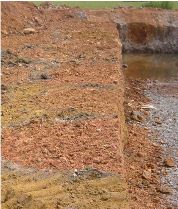
Figure 10. A vertical excavation for a hydraulic structure in improved peaty soil with heavy tamping. Crater outlines of peaty soil are visible on the horizontal ground on the bank of excavation
