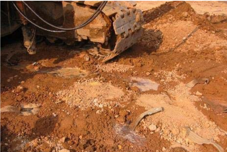
Figure 6. Prefabricated vertical (band) drains (FD) (100mm wide) at 1m centres near the crawler crane oozing water under pressure in the tamped peaty soil
