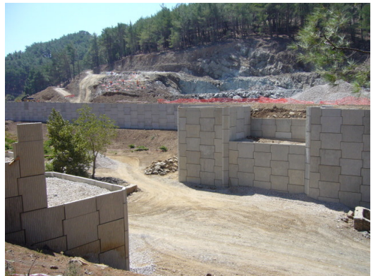
Figure 5. East and west bridge abutments leading on to retaining walls for mine process plant and offices
