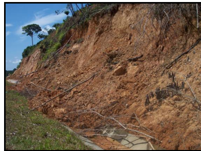
Photo 1 Sediments clogs side channels and culverts frequently.
