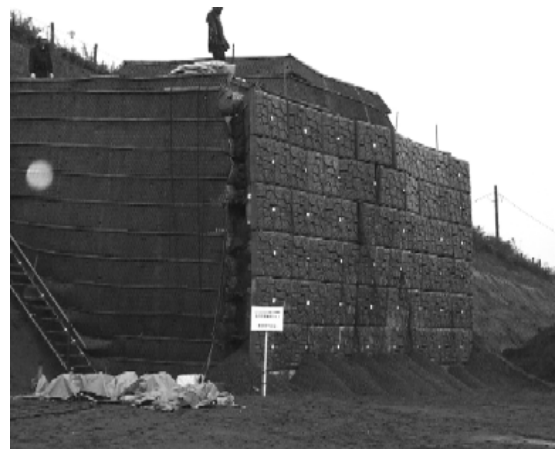
Figure 6. Wall surface deformation.
