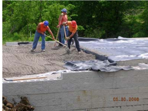
Figure 10. Integration of Approach Way for the Glenberg Bridge, next day after beam placement
