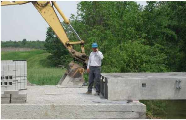
Figure 9. Placement of Concrete Box Beams Directly on the GRS Abutment (note absence of concrete footing)
