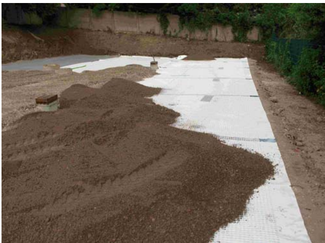
Figure 6. Covering of RDG and geogrid with the (reddish coloured) gravel base course material
