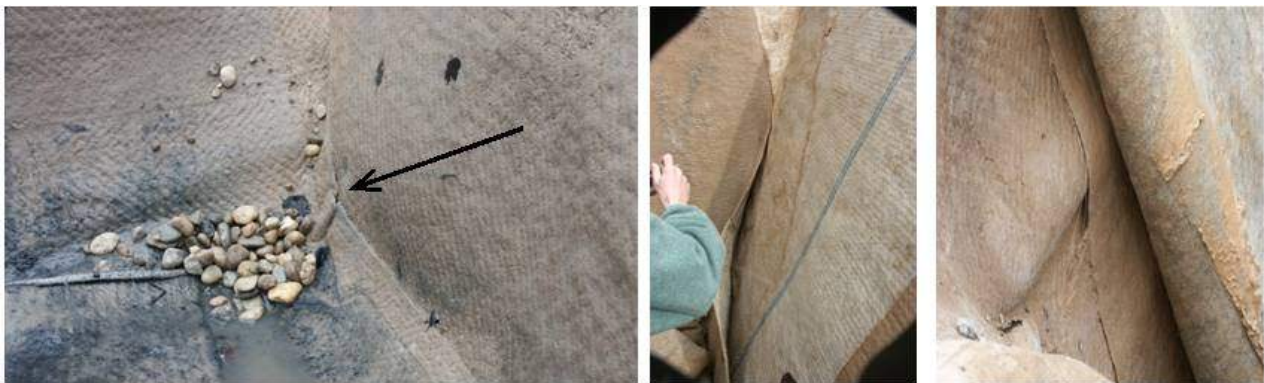
Figure 10. Installation errors: left: folding at the edge of the pit; centre: fabric on fabric; right, formation of a folding due to slip of the GCL
