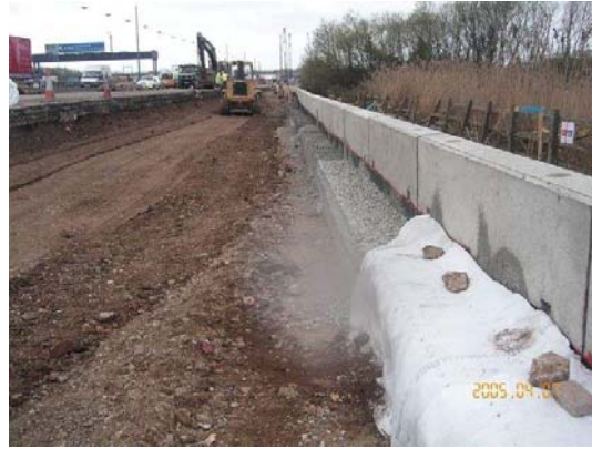
Figure 2. Geodrain at the back of an Earth Retaining Structure on the M25 London, UK
