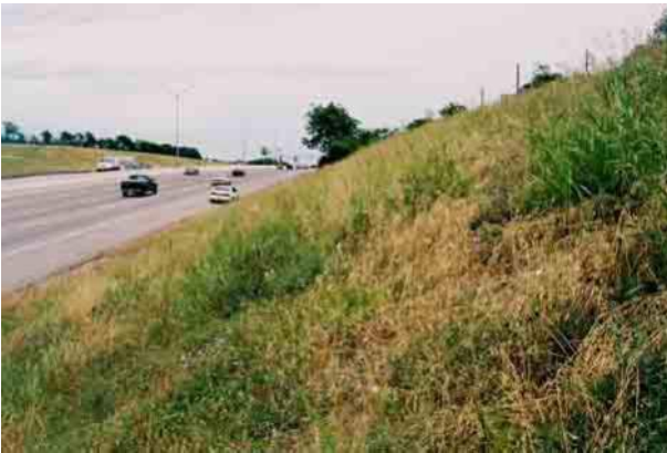
Figure 5. Slope failure repair at IH30, TX, USA around two years after completion.
