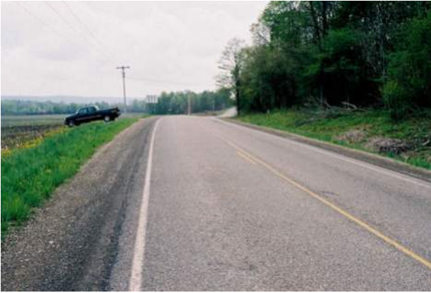
Figure 4. Road constructed over soft ground with a tyre bale foundation: Kabob Road, Stockton, Chautauqua County, NY, USA four years after construction.
