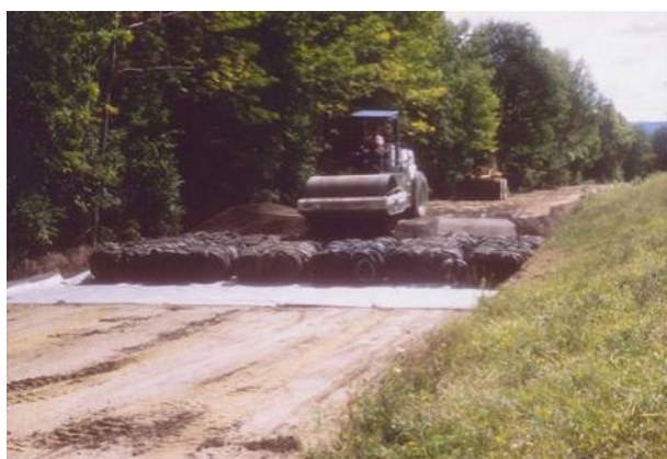
Figure 3. Road construction over soft ground using a tyre bale foundation: Condin Road, Ellery, NY, USA. (Courtesy of Chautauqua County Department of Public Facilities.)
