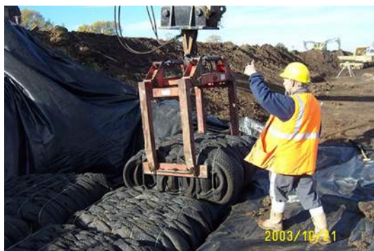
Figure 6. Placing tyre bales (using a pallet grab) within a wrapping of geosynthetic (© Environment Agency).
