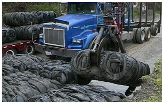
Figure 5. Placing tyre bales using a ‘loggers-clam’ (Courtesy, K Smith, Chautauqua Co. Dept. Public Facilities, NY).
