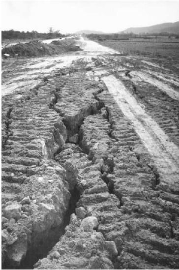
(a) Cracks on the embankment surface.
