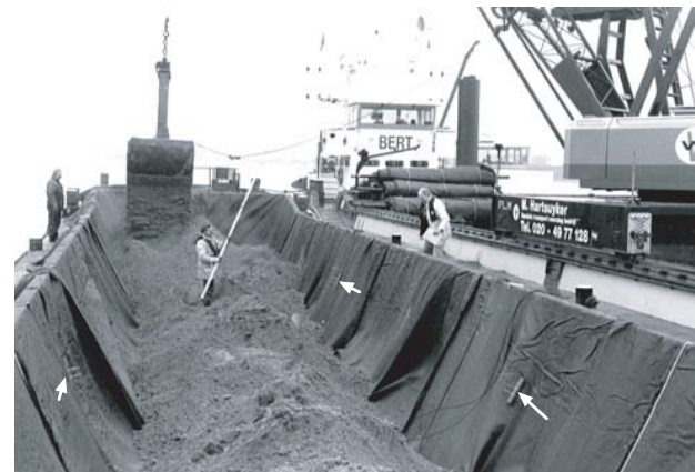
Figure 5. Overview split barge during installation of instrumentation. The arrows indicate the positions of the already installed strain gauges.
