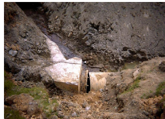
Figure 1. Damage to buried bend in the 1995 Hokkaido-Nansei-Oki Earthquake
