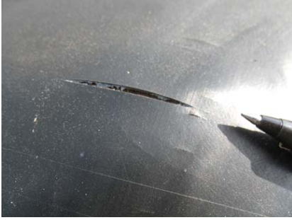
Figure 3 Long and short cracks on extrusion die lines at sub-grade stone protrusion
