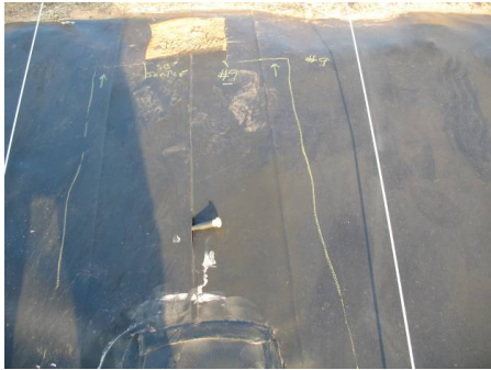
Figure 8 Cracked apex-down fold between two un-cracked apex-up folds (inside arrows).
