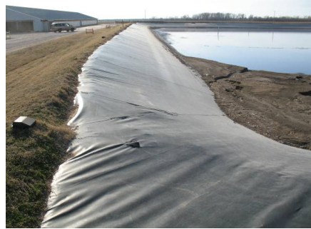
Figure 6 Taut liner at time of visit – temperature ~1°C.
