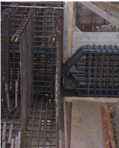
Figure 11. The beam connections were designed to transfer only horizontal and vertical forces.
