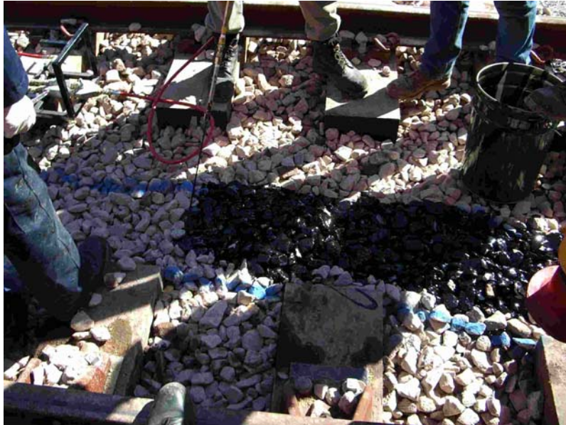
Figure 9. Formation of the upper polymer reinforcement at Tottenham South Junction, UK (upper reinforcement tied into lower reinforcement to form complete reinforced channel section)
