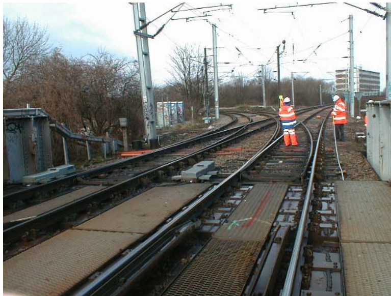
Figure 1. Example turnout from mainline with added bridge transition complication (Tottenham South Junction, UK)
