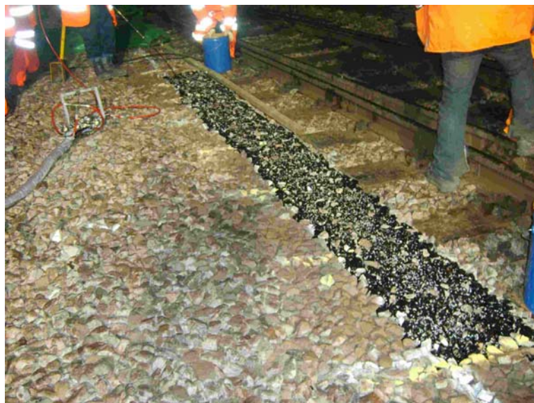
Figure 10. Formation of polymer side beams to increase passive resistance at Knighton Junction, UK
