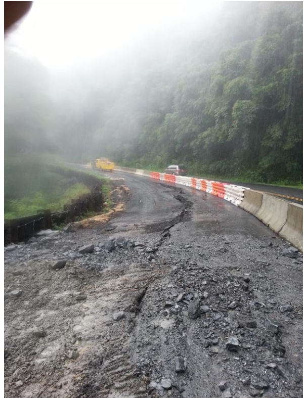
Figure 8: Failing Roadway Above Lagging Wall
