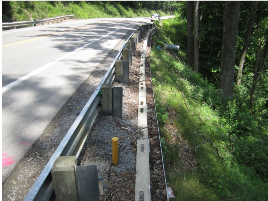
Figure 3: Failing Piling Wall
