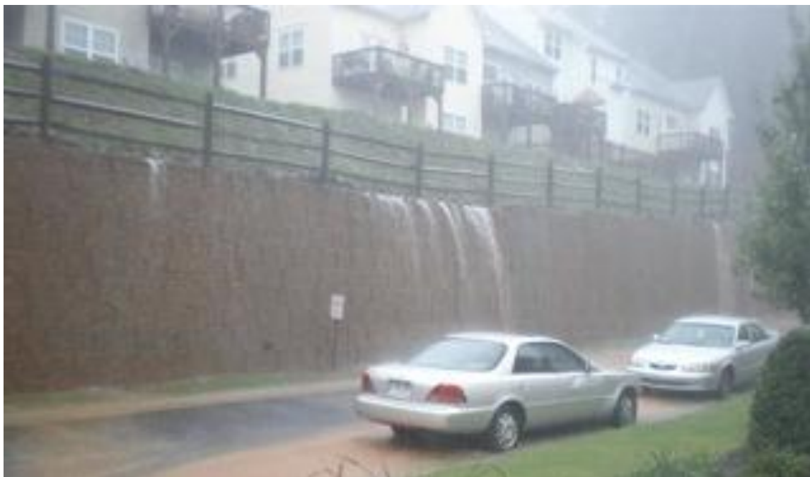
Figure 1: Inadequate Wall Drainage
