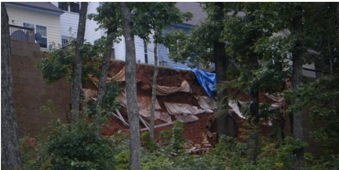
Figure 2: Failing Section of Wall
