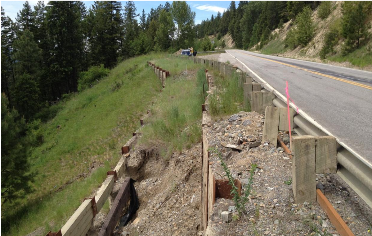
Figure 10: Failing Piling Walls
