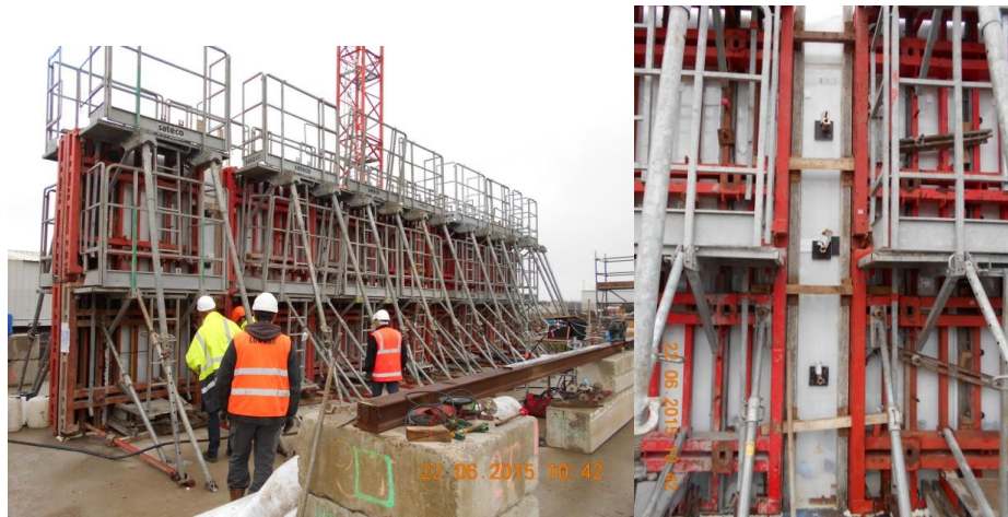
Figure 2. Mockup during the injection tests (left) and position of injectors on an injection profile (right)
