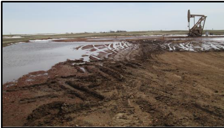
Figure 8. Well pad constructed with aggregate only, in need of maintenance.
