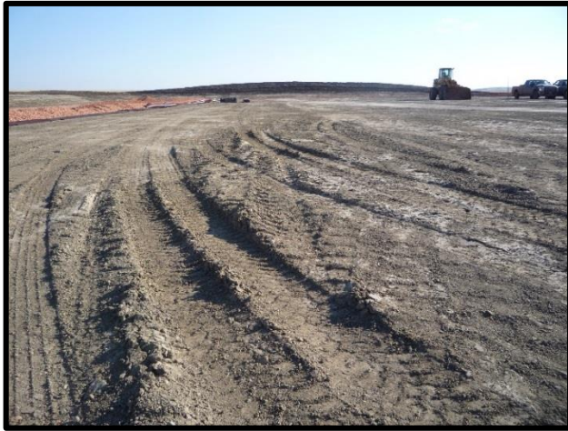
Figure 4. Soft subgrade condition requiring stabilization.
