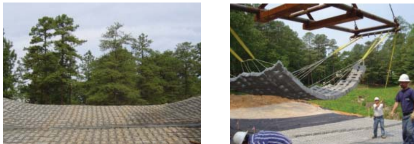
Fig. 27: Pre-fabricated articulating concrete block mats underneath by filter fabrics were used for suburban dam spillway and beach protection project (www.contechES.com, 2016)
