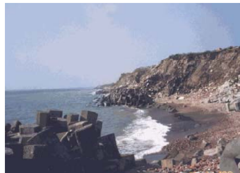
(b) Cliff coastline failure after typhoon attacks
