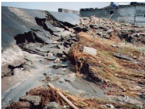
(a) Beach revetment protected coastline failure after Typhoon attacks
