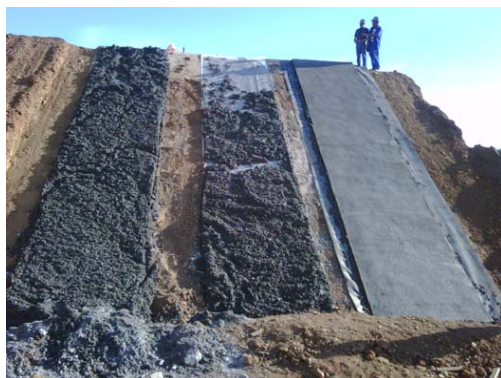
Figure 6. General aspect of geomembranes after concrete placement (from left to right – low asperity, smooth and high asperity geomembranes).
