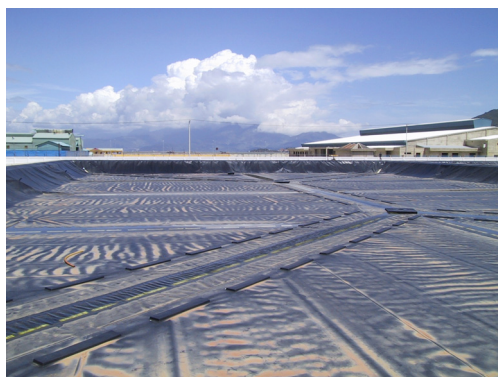
Figure 1. Wastewater container cover system.
