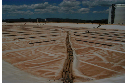
Figure 4. Caustic soda geotank in service.
