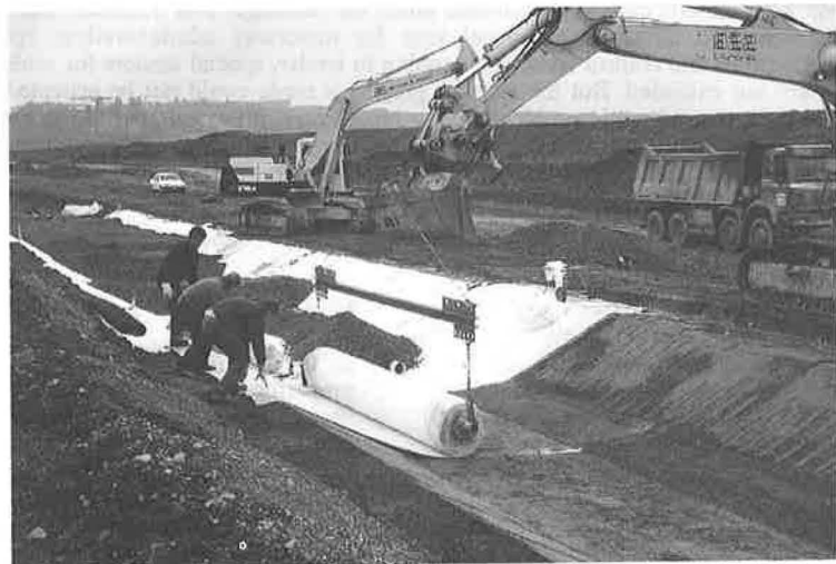
Figure 2. Installation of GCL in the further water protection zone in the area of the drainage pipe.
