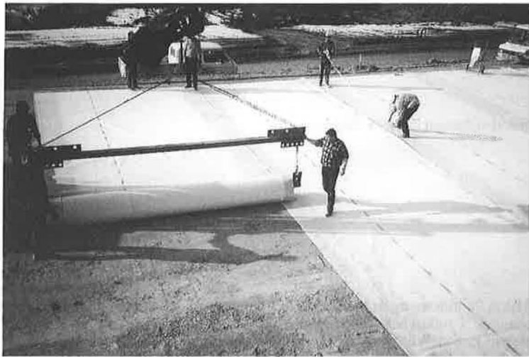
Figure 1. Installing GCL over a whole area in the immediate water protection zone at below zero temperatures and fixing the overlaps by a shear strip.
